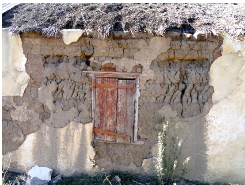
Photo 2 : Detail showing opgekleide wall with window insertion. Diagonal pattern formed by individual spadefuls of prepared clay, rows laid alternately. Top two rows probably added during a former roof repair.
