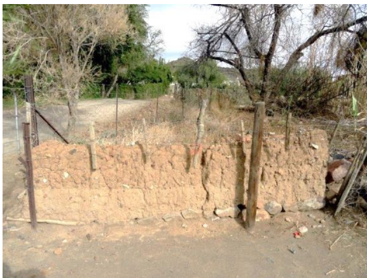
Photo 3: Last remnant of an opgekleide wall at entrance to Gay’s dairy. Note crude stone foundation.
